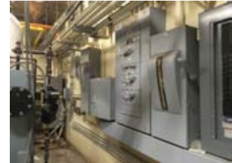
Single Phase Electric Service
