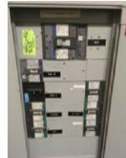
Three Phase Electric Service
