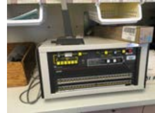
Existing Intercom Head-End
