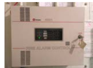
Fire Alarm Control Panel
